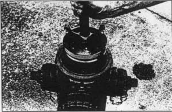
23. Reversing above procedure, reinstall valve assembly, fully threading it into the subseat. You may pull up on rod, closing valve, and opening auxiliary valves to pressurize the elbow and check for any leaks.
